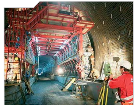
Setting out of the framework for the inner shell of a tunnel
