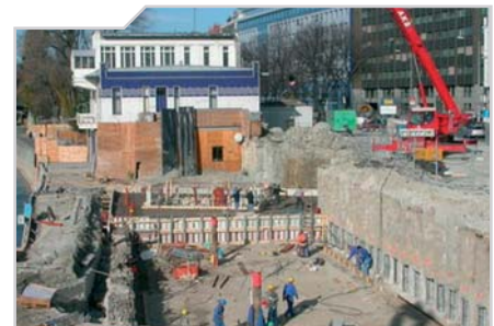
Setting out of a foundation and of bored piles on the surface
