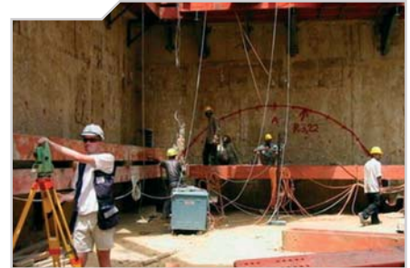
Setting out of the profile for a tunnel in the starting shaft
