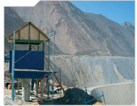
Measuring station for monitoring a sliding slope in a mine
