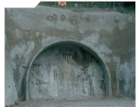
Permanent profil checks guarantee an optimised excavation profile for all construction phases
