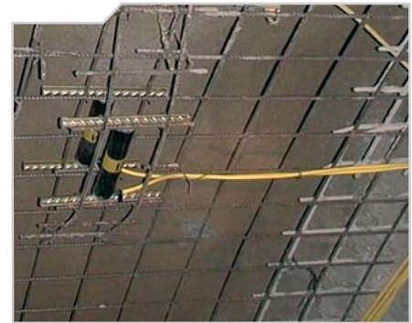
Strainmeters installed in pairs
