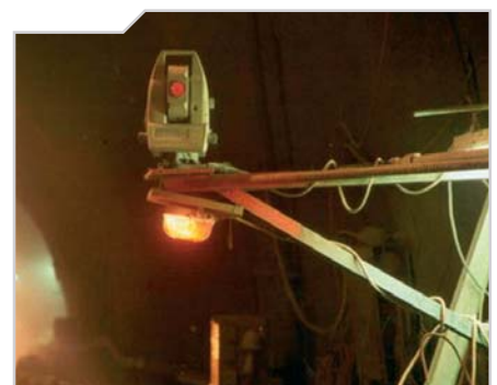
Totalstation as part of a motor laser system on the side wall
