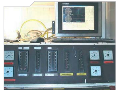
Control computer in driver's cab of a TBM
