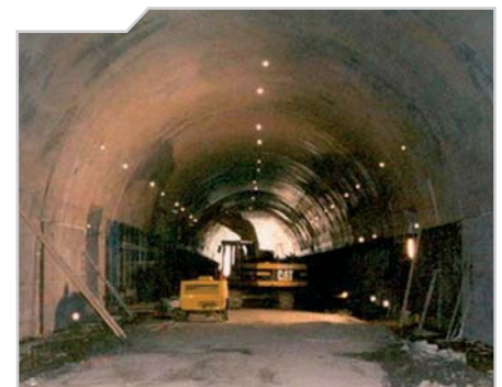
Monitoring sections with Birefle-targets for displacement measurements in the inner lining of a tunnel
