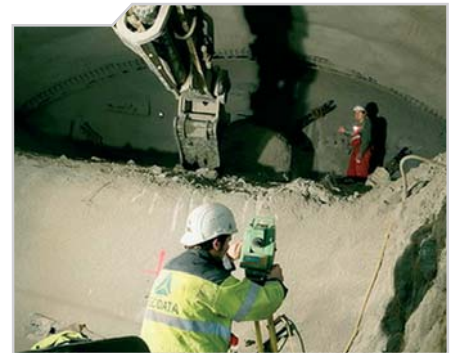
Surveying in the side wall gallery of the Lainzer tunnel in Vienna
