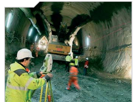
Heading control of side-wall drifts during construction of the Lainzer Tunnel in Vienna
